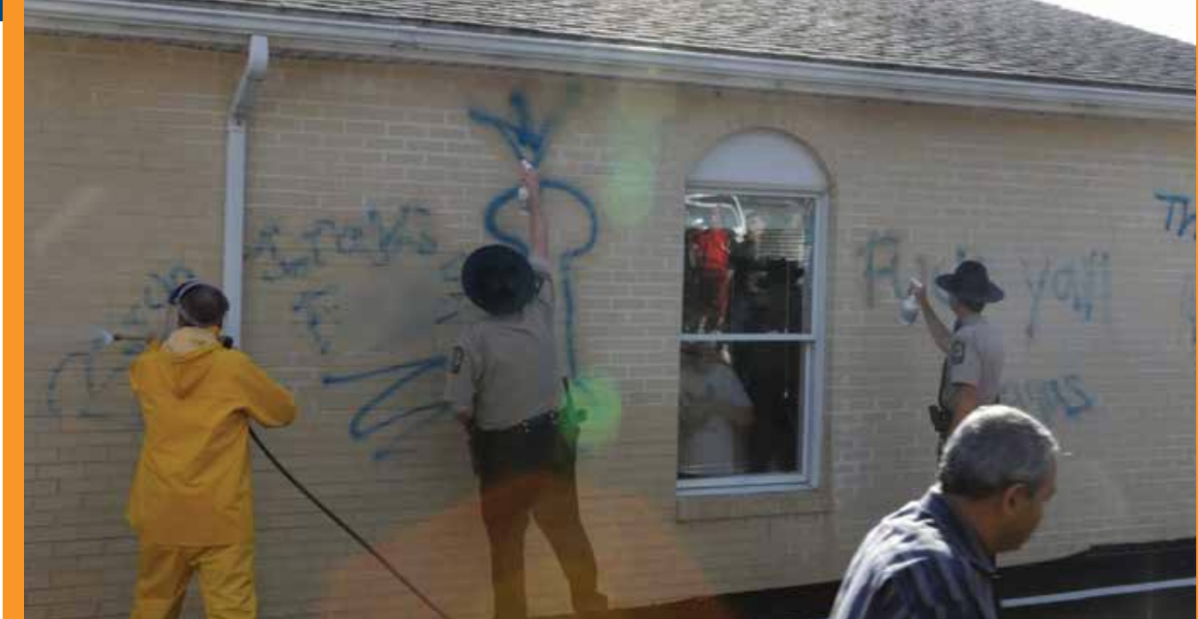
Hate graffiti being cleaned from the Islamic Center of the Shenandoah Valley in Harrisonburg, Va.
