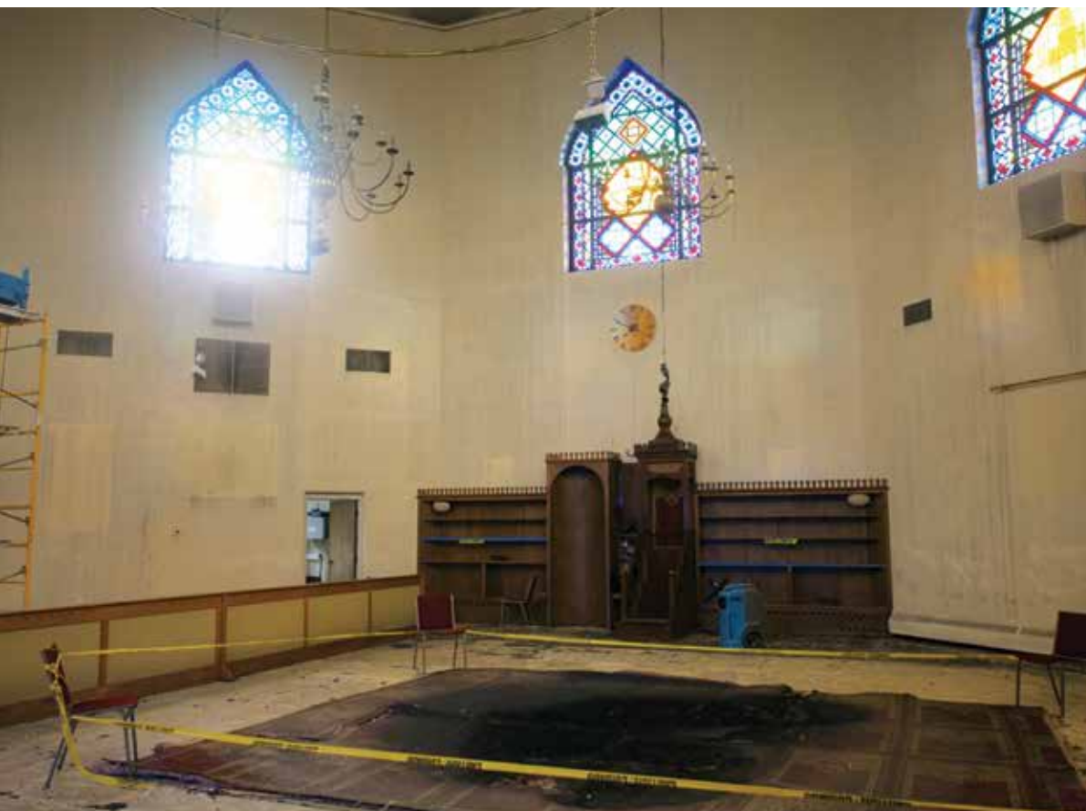
Arson-damaged interior of the Islamic Center of Greater Toledo in Toledo, Ohio.
